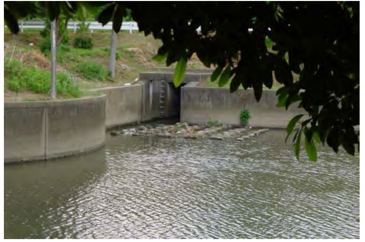
①家下川－承水溝の段差
