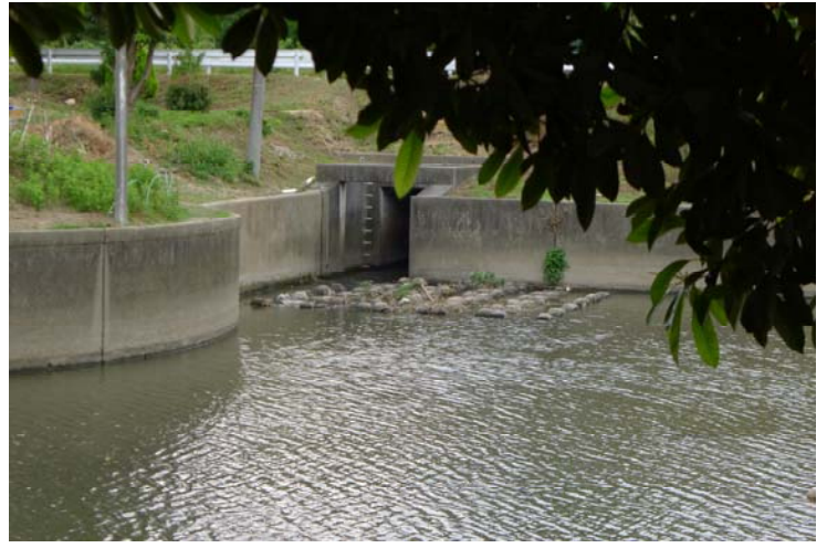
①家下川－承水溝の段差
