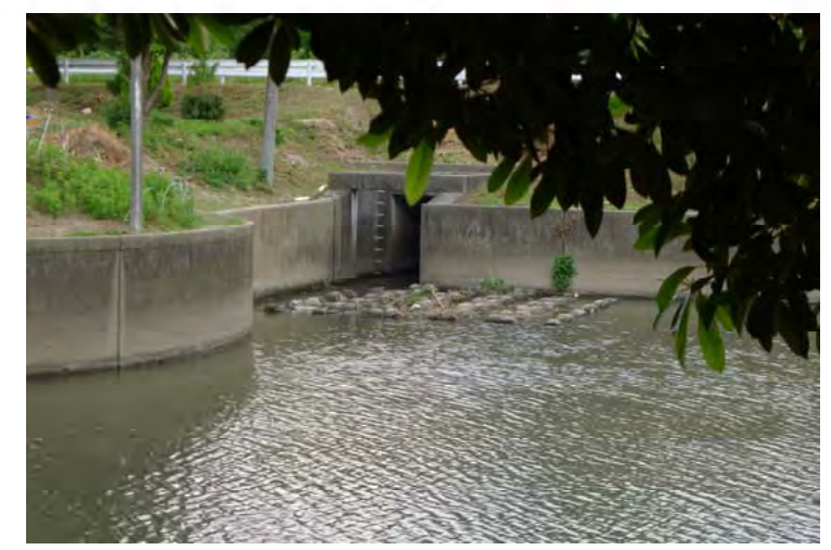
①家下川－承水溝の段差
