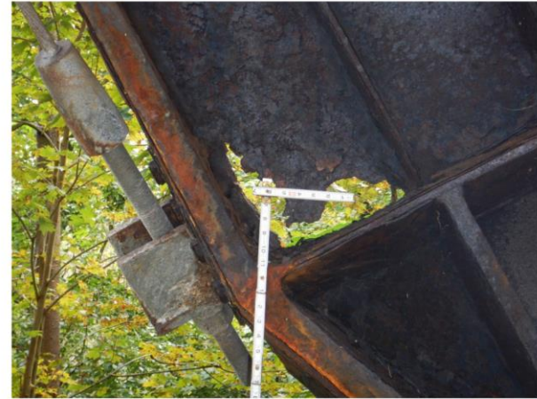
BENT 1, RIGHT FRAME LEG Note: 100% section loss in web
