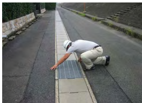
①高潮堤防の川裏排水側溝
