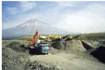
The removal of rocks and sifting out of pebbles from deposited sediment
